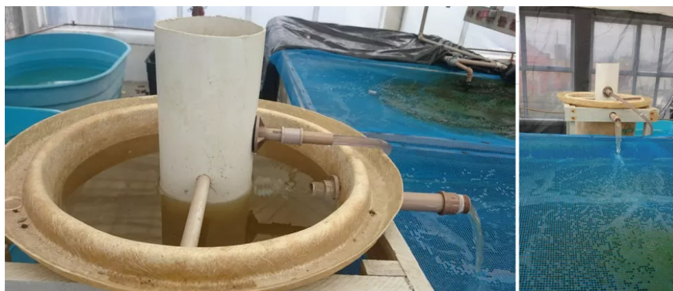
View of the solids removal system in the experimental setup.
