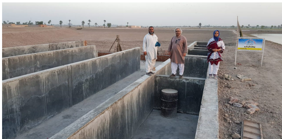
Views of the raceways, quiescent zone (QZ) area and waste tanks.
