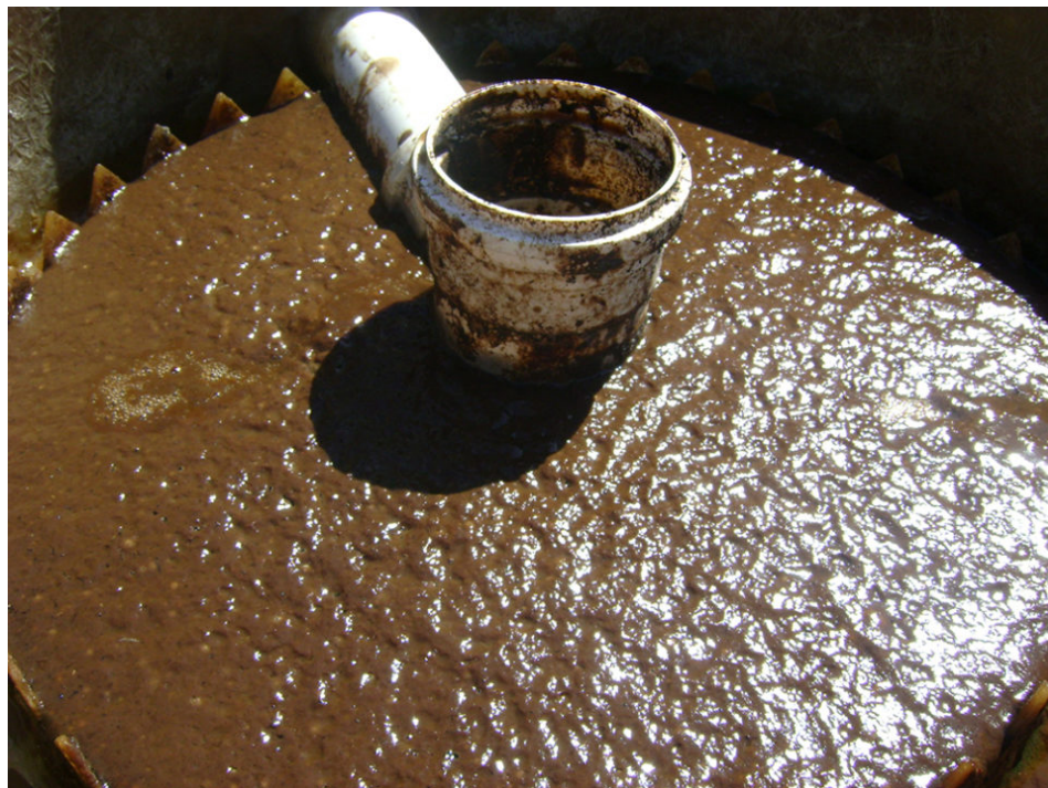
Biofloc in the settling chamber of the activated sludge system.
